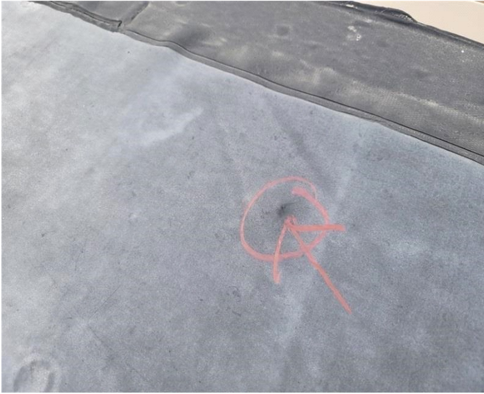
F-102 Field Membrane - puncture/Hole/tear # 3
