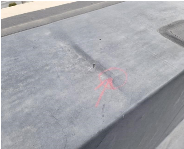
F-102 Field Membrane - puncture/Hole/tear # 1
