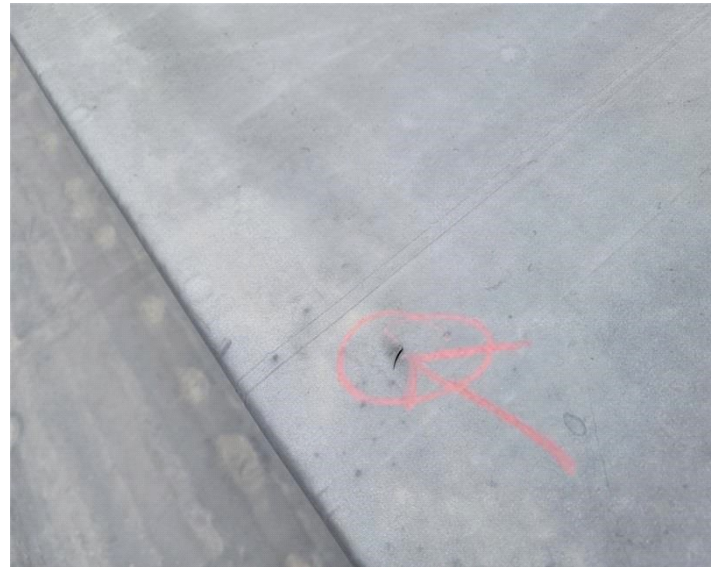
F-102 Field Membrane - puncture/Hole/tear # 2
